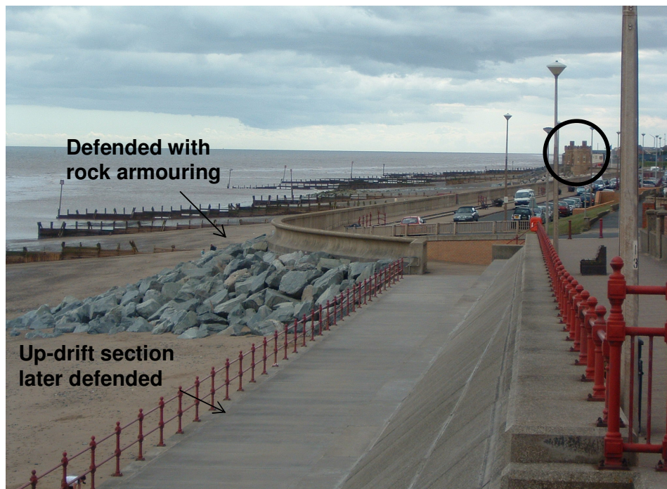
Figure 7.5b – Withernsea North Promenade defences and rock armouring in 2006. For reference, the circle illustrates the same building on Figure 7.5a. Photograph taken 10th August 2006.
