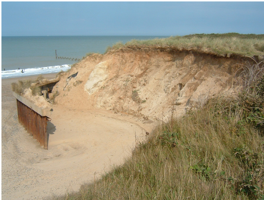
Figure 6.12 - Up-drift defence outflanking at Happisburgh. This defence is situated at the down-drift end of the set-back, thereby creating an 'initial groyne effect'. Drift direction is from left to right of the figure. Photograph taken 16 th August 2006.
