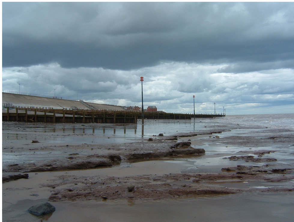
Figure 4.38 – Wooden groynes and a seawall at Withernsea. At the seaward end of the groynes, there is very little sediment and the shore platform is exposed. Photograph taken 10 th August 2006.
