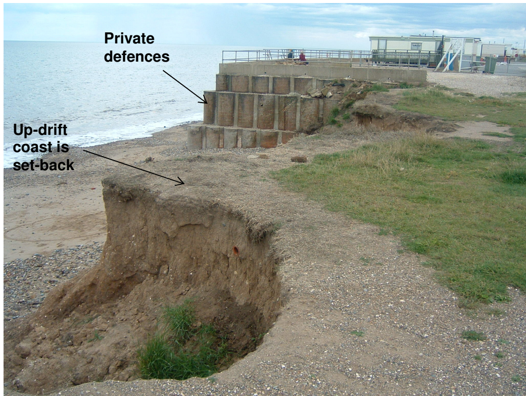
Figure 7.7 - Private defences at Ulrome, Holderness. A seawall does not retain a beach. The up-drift coastline is set-back, creating an 'initial groyne effect' and allowing the defences to form a small headland. Photograph taken 10 th August 2006.
