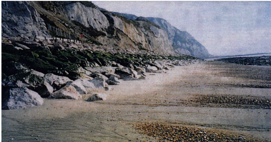
Figure 2.6 - A rock armoured revetment at Folkestone, Kent (photograph taken in 2002, courtesy of Andrew Pearce).
