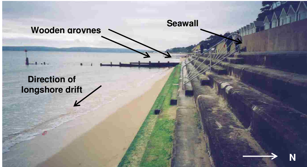
Figure 2.5 - Groynes and a seawall at Poole Bay, Dorset prior to beach replenishment in 2006-2007. Longshore drift direction is coming out of the photograph, parallel to the seawall. Note handrail for scale (photograph taken 5 th December 2004 by Andrew Pearce).
