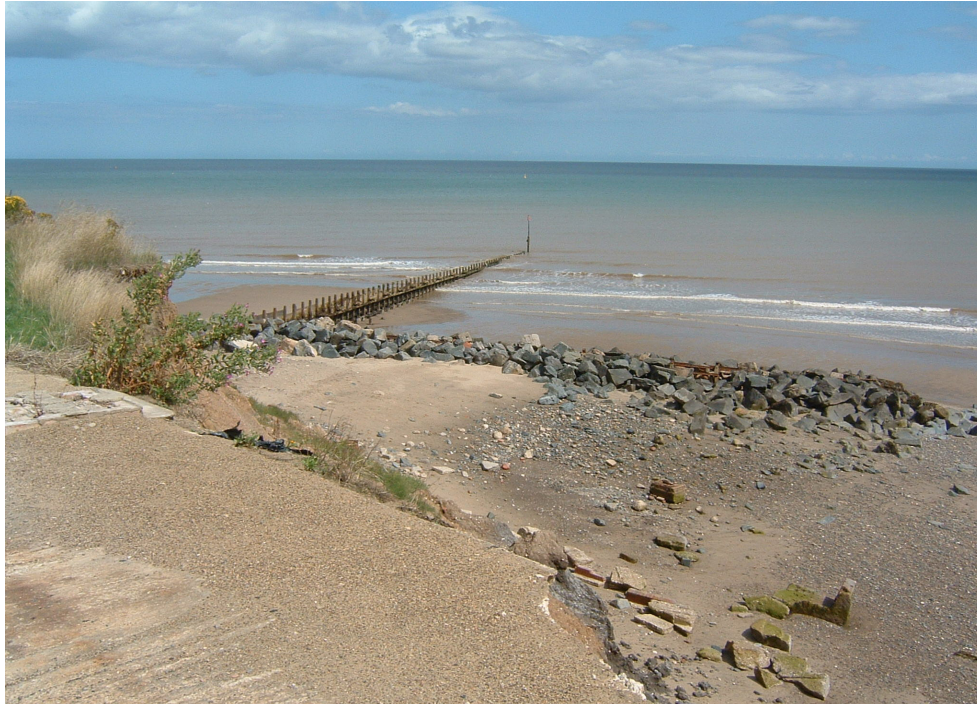
Figure 4.20 – The outflanking structure at Hornsea. Composed of rock armouring, this T-shaped structure is not connected to the seawall, allowing outflanking and erosion to continue behind the structure. Photograph taken 9 th August 2006.
