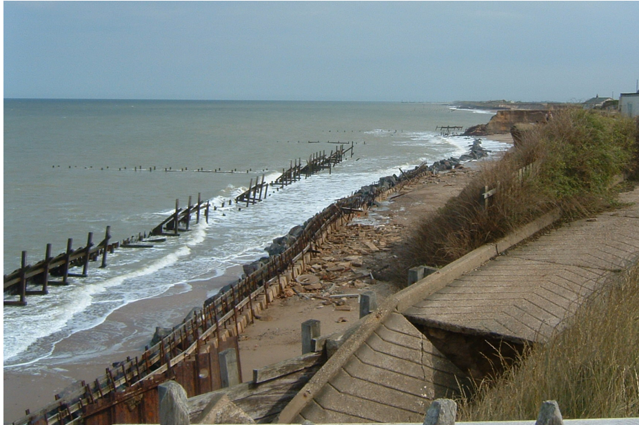
Figure 6.13 – Abandoned groynes and revetments at Happisburgh. Some of these defences are not visible when it is high tide, so pose a danger. Other abandoned defences are much more subtle, and protrude out of the beach by only a few centimetres. Photograph taken 16 th August 2006.
