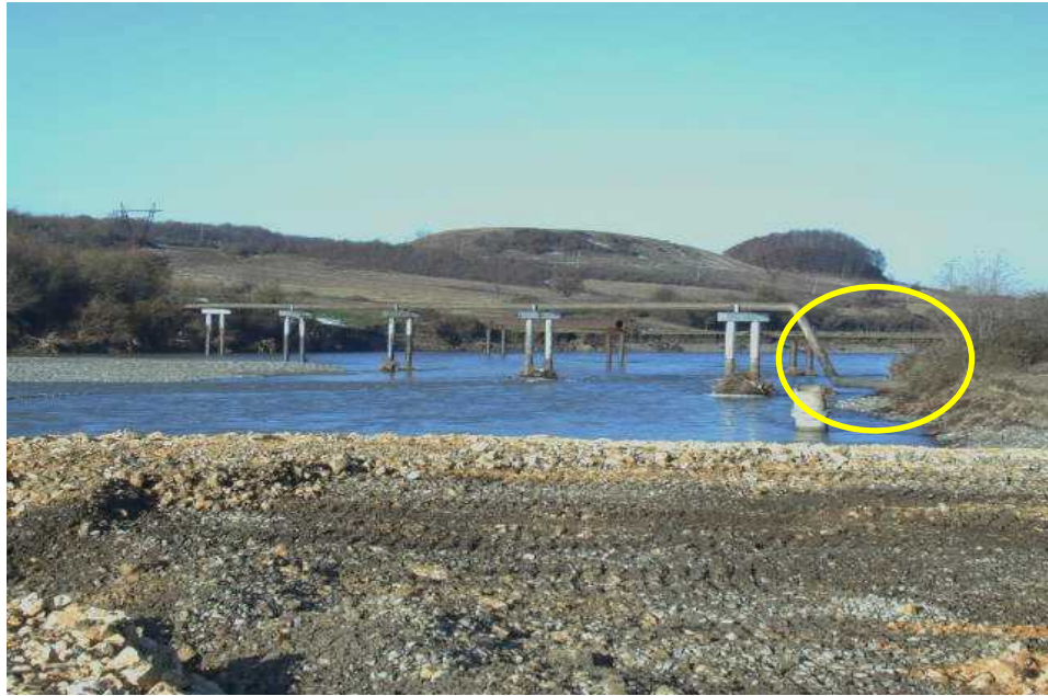
Figure 1.1: Aerial pipeline exposure due to bank erosion, the Kvirila River near to Zestaphoni, Georgia. Photograph has been taken in 1999 by Prof. P.A. Carling.
