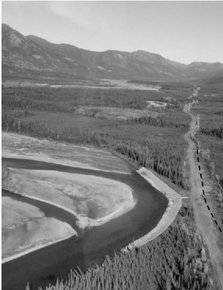
Figure 1.3: Riprap revetment constructed to prevent bank erosion in a reach of the Middle Fork Koyukuk River, Trans Alaska Pipeline, Alaska. The dashed line locates a buried pipeline. Date of photograph is September 2001, from Veldman and Ferrell, 2002.
