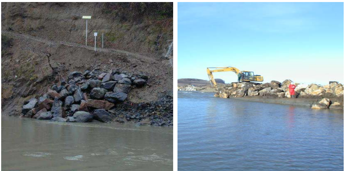
Figure 1.2: Riprap revetment constructed to prevent bank erosion at buried pipeline crossings, Georgia. Photographs have been taken in 1999 by Prof. P.A. Carling.
