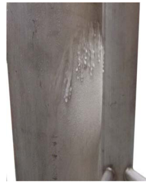
Figure 8: Ice accretion on the outside of the pipe by the test valve
