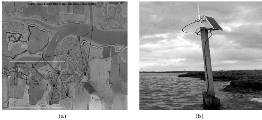
Fig. 1. (a) The deployed FLOODNET system in the River Crouch, East Essex in eastern England. (b) A FLOODNET node on site.
