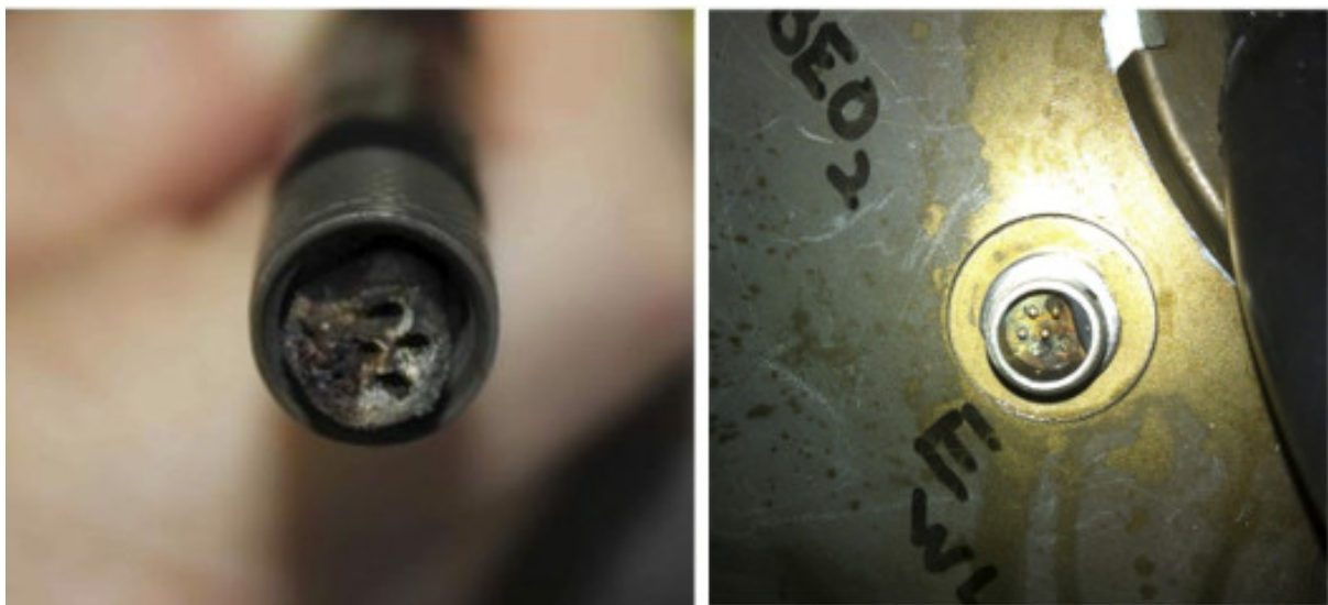
Figure 36: (Left) Photograph of melted plug after blown cable. (Right) Photograph of partially corroded socket.
