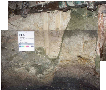
Figure 4 Shear surface exposed in a trial pit
