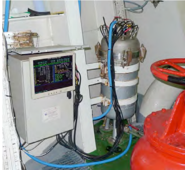
Figure 2.1. The SNOMS flow through tank and data unit installed on the MV Pacific Celebes , in the ship's machinery space.
