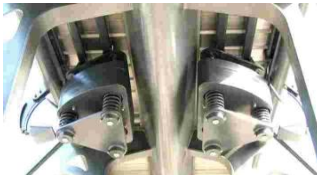
Figure 1.2 Multiple dynamic vibration absorbers are installed to a bridge [9].
