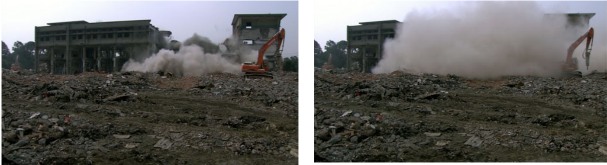
Figs. 3 and 4: A factory building collapsing in 24 City
