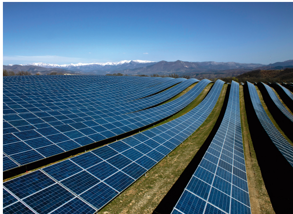
Figure 1.3: A photovoltaic power station [18]
