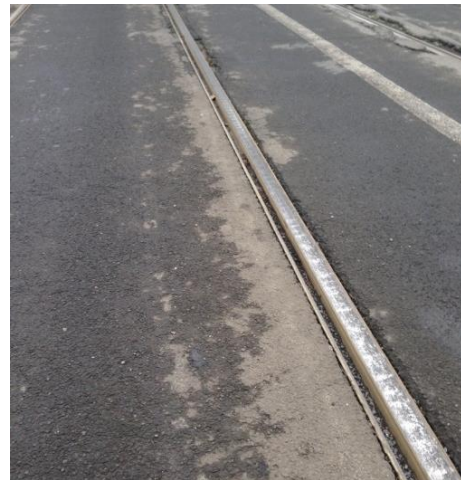
Figure 1. Corrugated rail R, relating a straight section of the right track of a bidirectional line.
