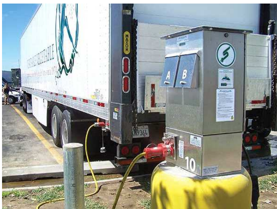
(a) Electrified Parking Space
