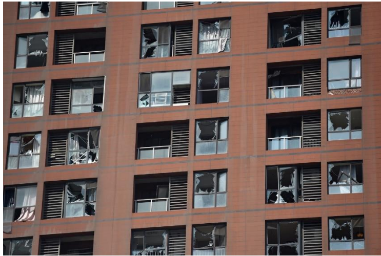
Figure 1. Damage to windows in a residential block near to the Tianjin explosion[8].
