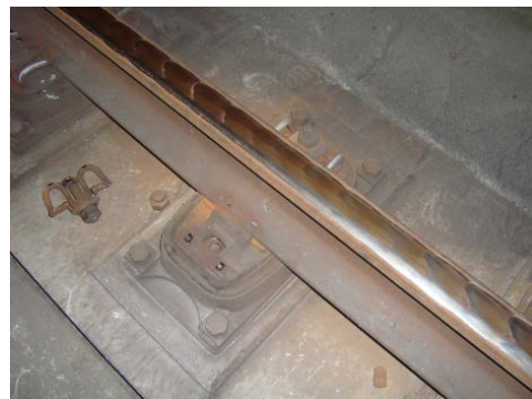
Figure 1. Corrugation exhibited on the rail with Egg fastener. Note the broken rail fastener
