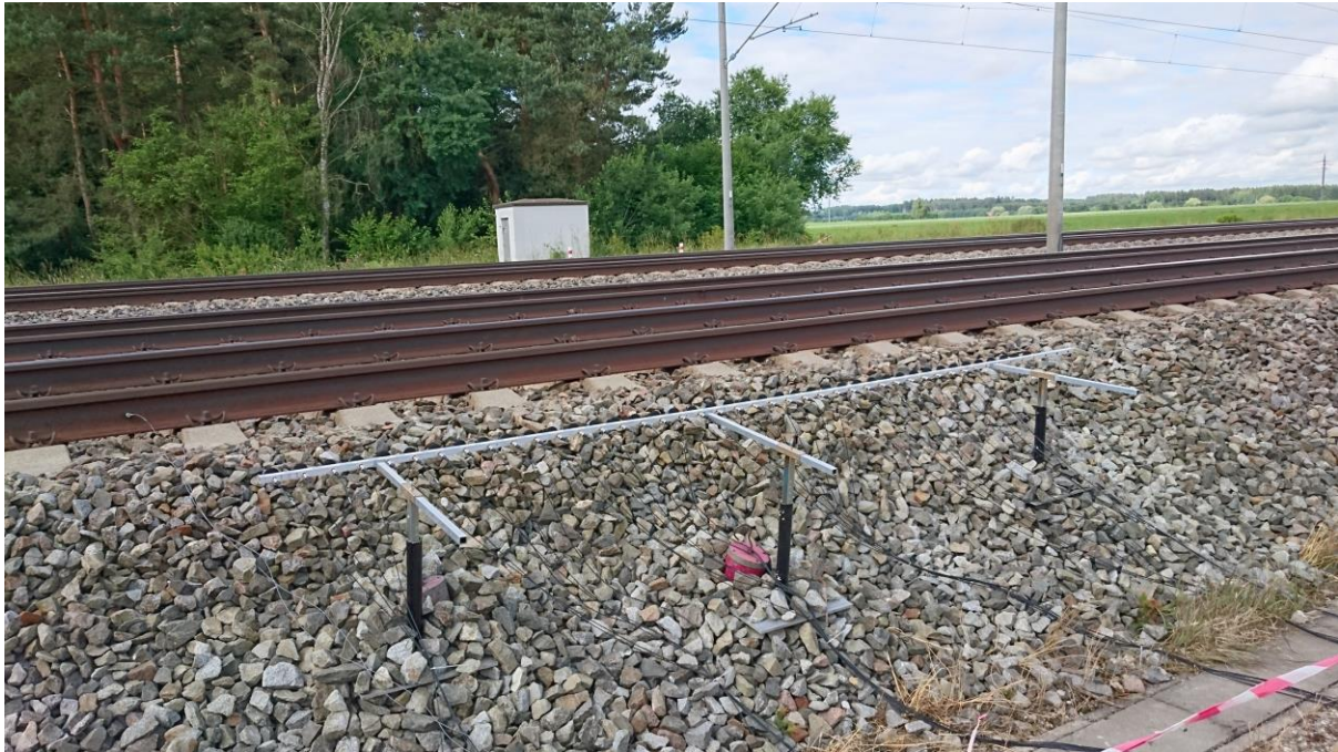
Figure 10. Photograph of the linear microphone array setup at the WSE site.
