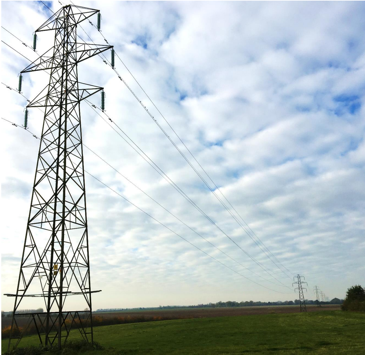
Figure 7. 132-275 kV high voltage transmission powerlines crossing a natural landscape in the United Kingdom
