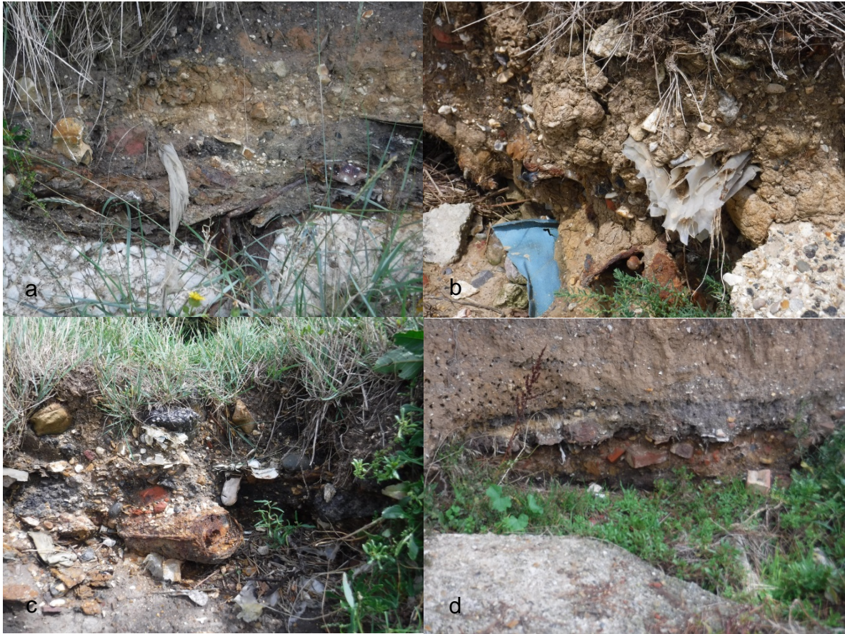
Figure 3: Visible waste in the sea wall/landfill frontage at the Wicor Cams study site (11 August 2017)..
