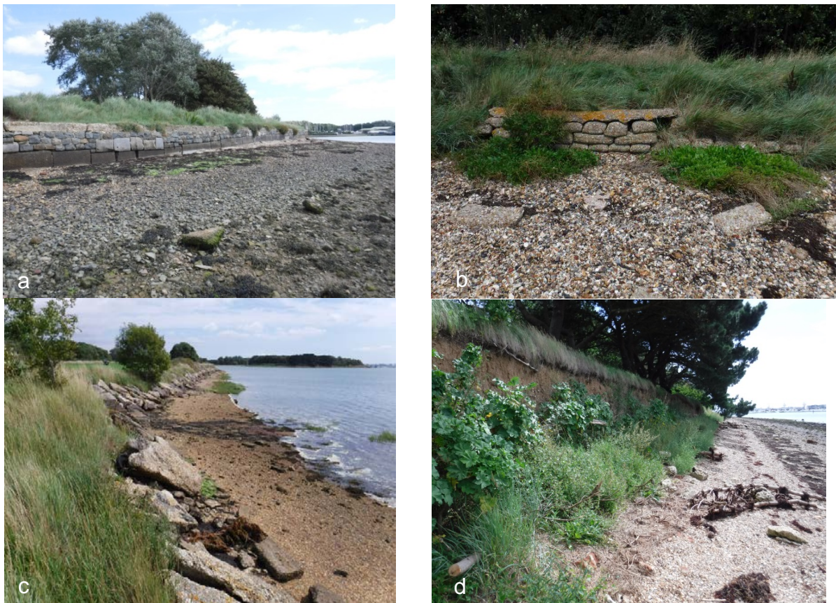
Figure 2: The sea wall and frontage to the landfill sites at the Wicor Cams study site (11 August 2017).
