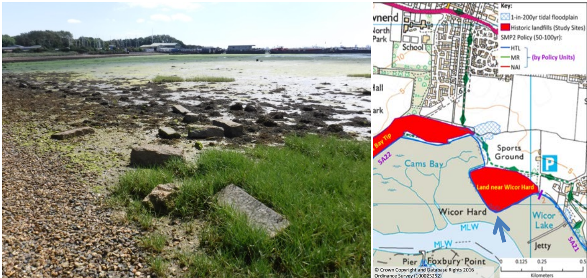
Figure 4: Erosion of the sea wall at the Wicor Cams study site (11 August 2017). The arrow on the map shows the location of stone blocks from the sea wall which are now on the foreshore.
