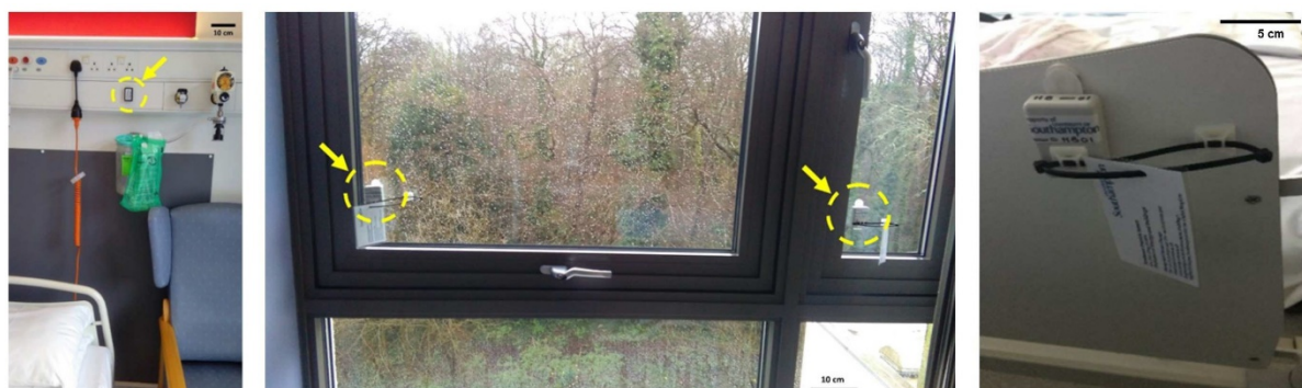
(a) TEMP: Air temperature and relative humidity sensors in the case study ward.
