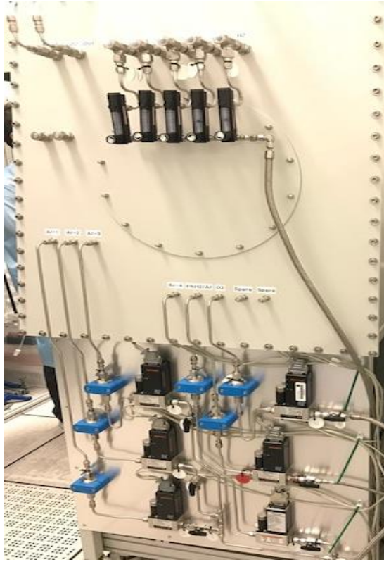
Figure 3.3 Gas flow control panel with all MFC's.
