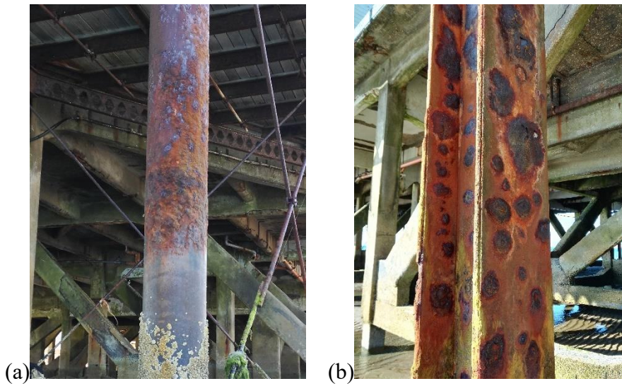
Figure 1 Locally pitted steel columns under marine environment [22]. (a) Tubular section; (b) H section.
