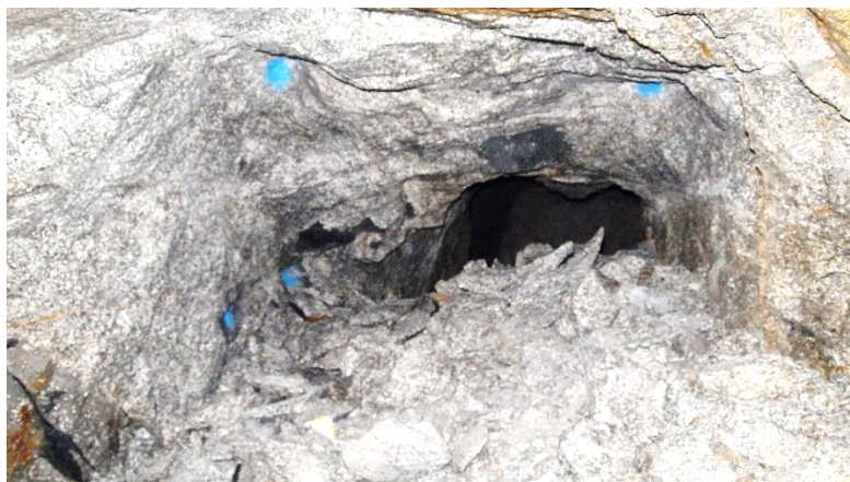
Figure 70 Cross cut expansion post blast with the remnant of the blast holes marked by blue paint
