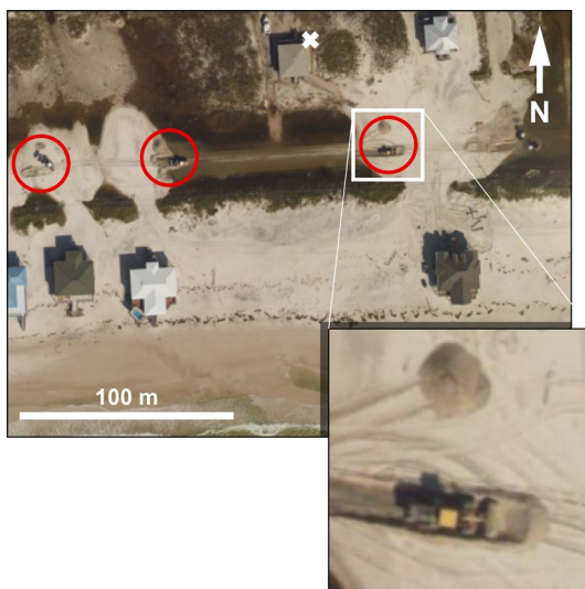
Figure 1. Excavators (circled and detailed) clearing washover sand from the main road along Dauphin Island, Alabama, October, 10 2017, 2 days after Hurricane Nate. (Location marker x: 30°15'03"N, 88°10'77"W.) Image courtesy of National Oceanic and Atmospheric Administration (NOAA).
