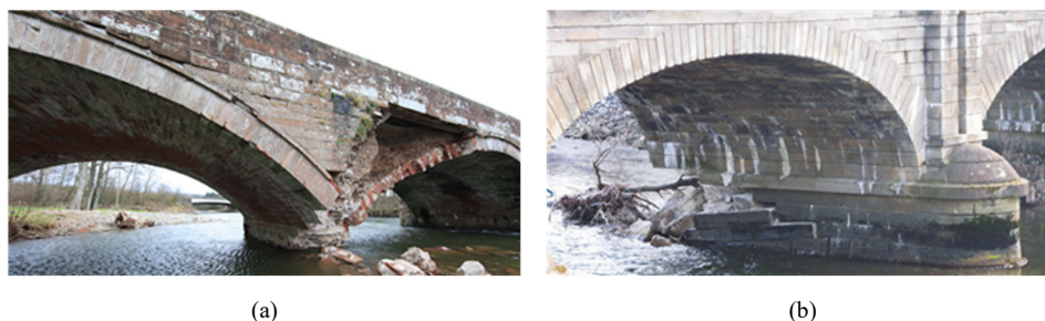
185 Figure 2. Damage of Brougham Old Bridge (a) and of Calva bridge (b), typical of many masonry arch bridges subjected to scour (Source: Cumbria Council County for (a) and Bill Harvey for (b)).
