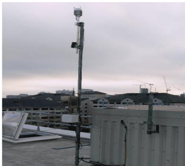
Figure 3.2 Weather station at substation of Transformer A.
