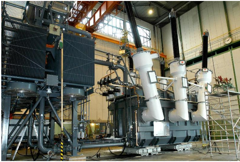
Figure 1.1 A large power transformer, used with permission from National Grid Electricity Transmission
