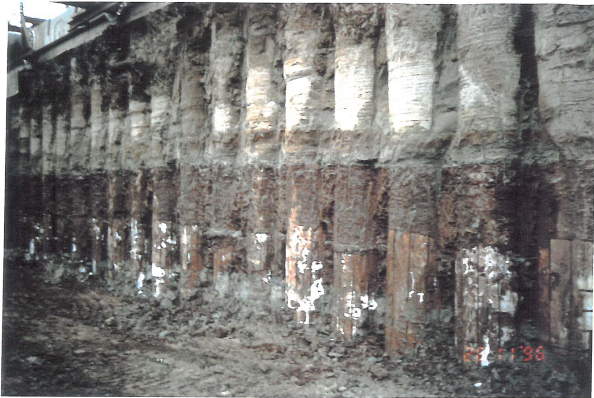
Figure 3.4. Weak rock debris clinging to face of the piles at the instrumented wall
