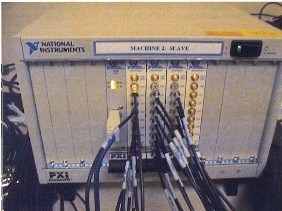
Figure 5.8 PXI1000B chassis with NI4472 data acquisition cards.
