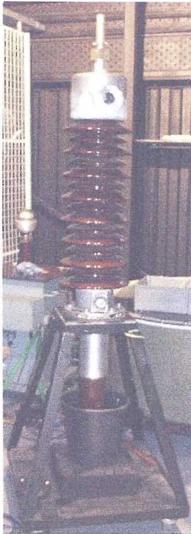
Photo 3.1, The 60kV Bushing
