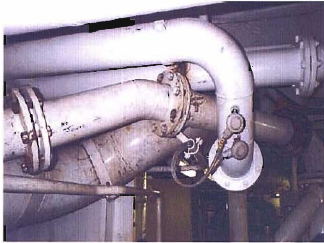
FIGURE 10.2: Example of pipework in an engine room
