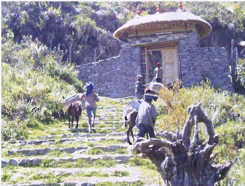
Figure 37: Transport of stones by the students of Ankober for the renovation of the Safe House building, June 2003.
