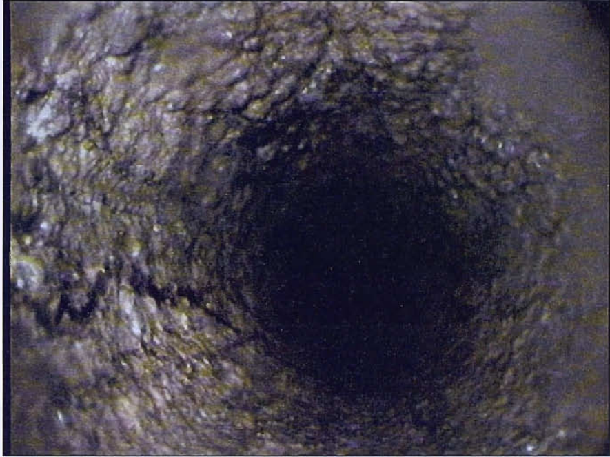
Figure 4.2. Probable calcium carbonate precipitation on well casing above the leachate level. Well internal diameter approximately 170 mm (well 207, Warnham landfill)
