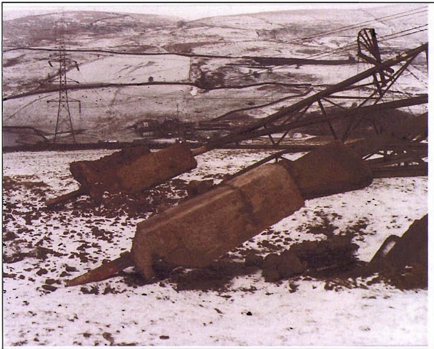
(b) Tensile failure of an un-cleated footing stub
