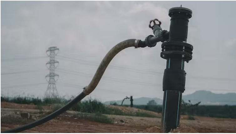
Methane gas pipes can collect emissions from landfills. Aaronwky/Shutterstock
