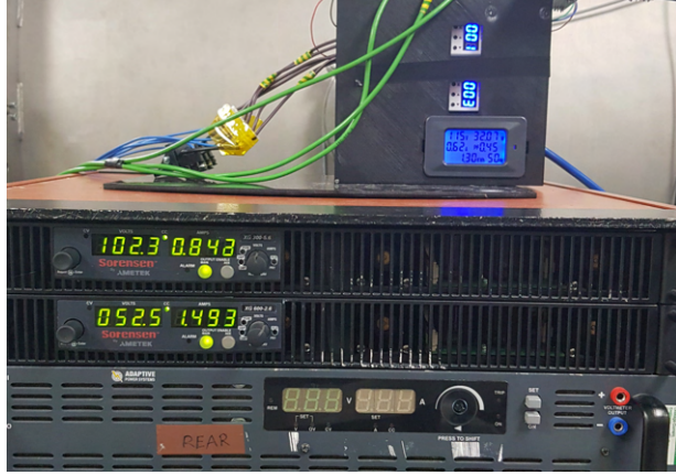
Fig. 10 Mark 3 PSDS control system (top) and thruster DC power supply (bottom).
