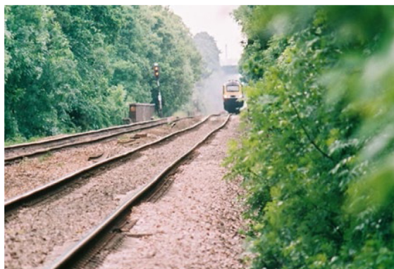
Fig. 4. Differential settlements in the trackbed, photograph courtesy of Graham Birch, Network Rail.
