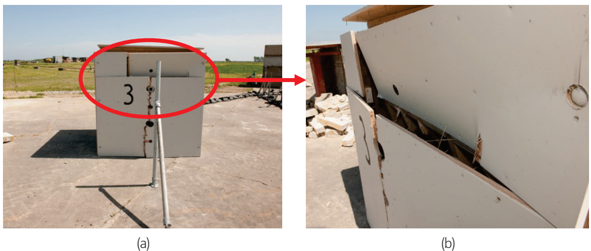
Figure 6.5: Post-trial images of timber structure, 14.25m: (a) Frontal damage; (b) Magnified view of damage.
