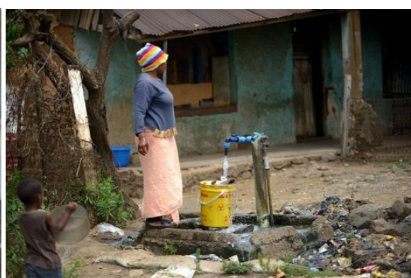
Figure 2-4: Public standpipe in South Africa (Source: Mabaso, 2016)
