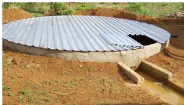
Figure 2-10: Underground concrete storage tank (Source: Mwenge and Taigbenu, 2011)
