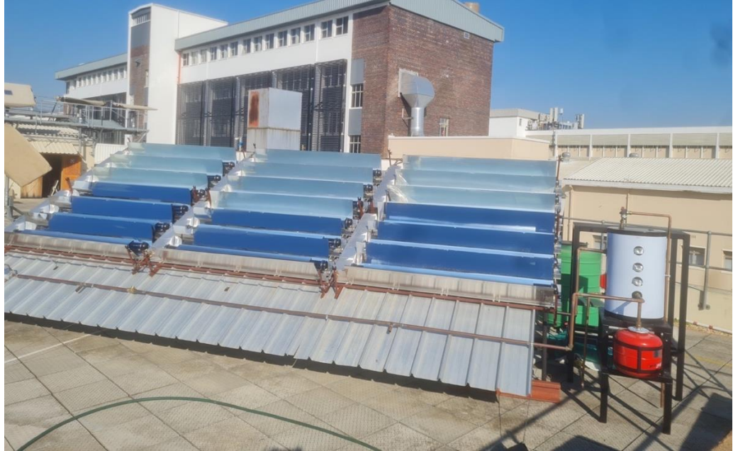
Figure 5-2 Photograph of combined system solar collectors and boiler cylinder built on laboratory roof at the University of Stellenbosch. Reproduced with permission from Dr Michael Owen from University of Stellenbosch Solar Thermal Energy Research Group.
