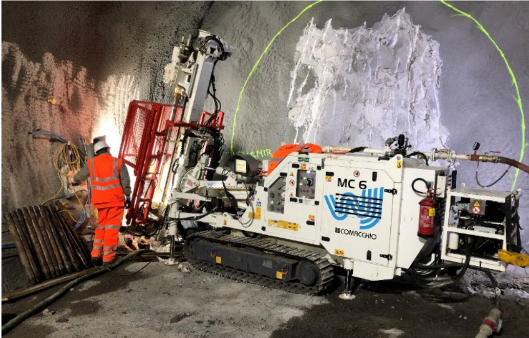
Figure 5: Installation of in-tunnel wellpoints in a tunnel heading (constructed by SEM/SCL methods) using an electrically driven drilling rig (Image courtesy of WJ Group)
