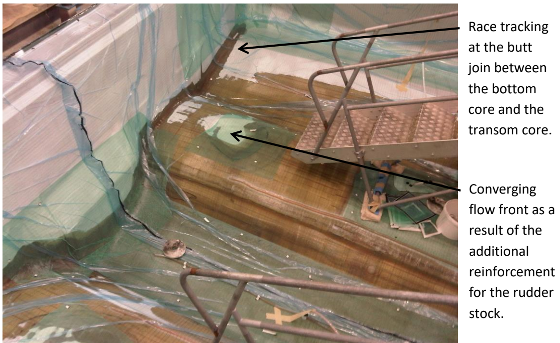
Figure 11: PYI M40 infusion demonstrating the effects of non-uniform preform permeability resulting in flow front convergence at the rudder stock and race tracking due to bag bridging at the hull transom join.
