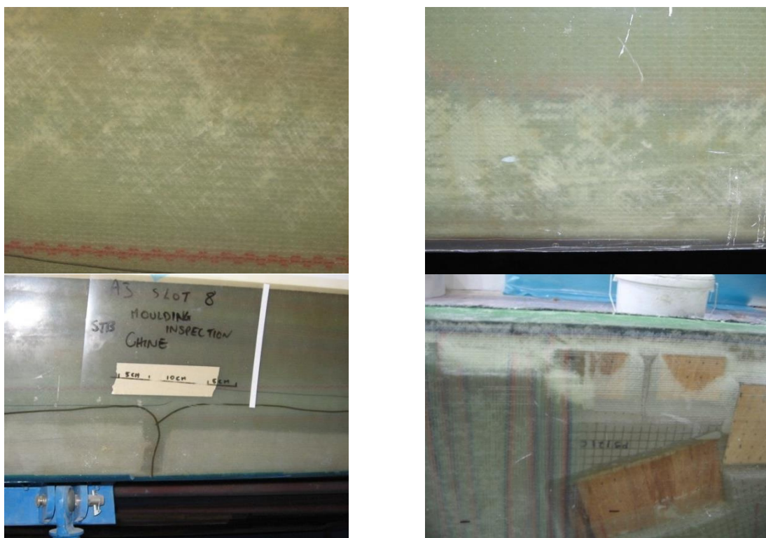
Figure 2: Void Defects in VARI components at PYI.
