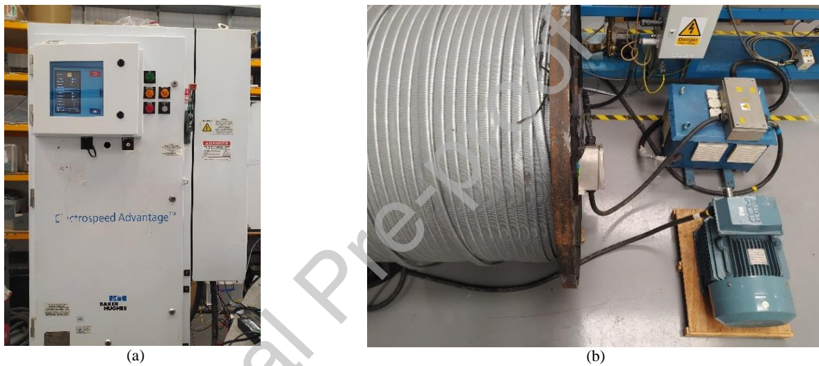
Fig. 9. Photographs of (a) VSD, and (b) cable, transformer and motor of the experimental setup.
