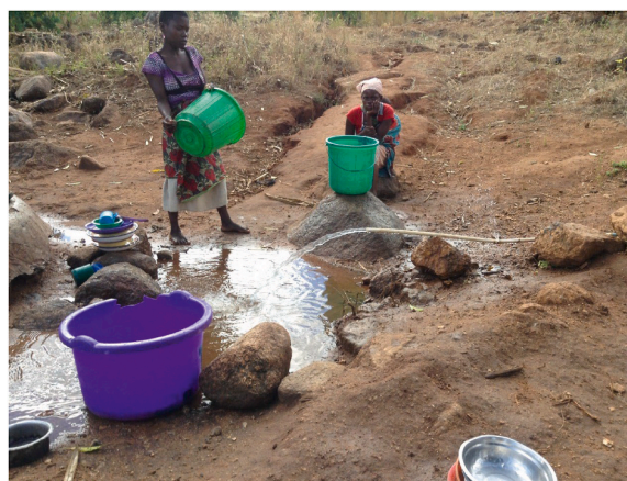
Fig. 8. Damaged pipe in Mtuluma (Source: Matthews Tsirizeni, LEAD).
