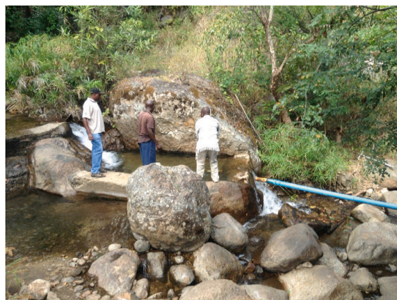
Fig. 9. One of the intake structures in Mtuluma (Source: Matthews Tsirizeni, LEAD).
