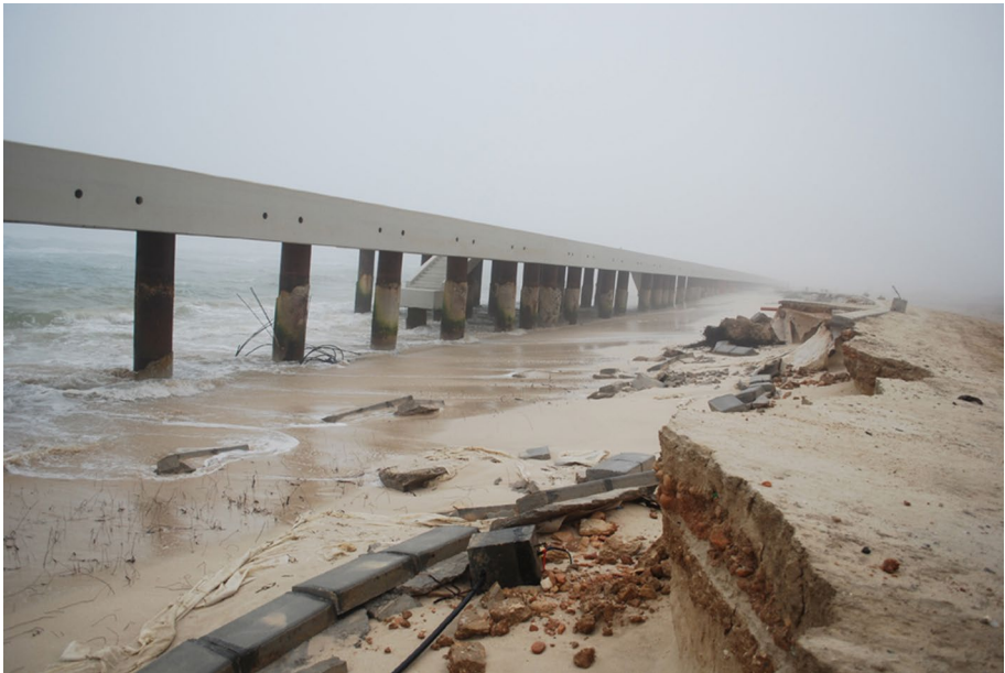
Fig. 7 Picture showing erosion off the coast of Al-Baleed near the pedestrian bridge in 2013 (taken by and used with the permission of Tom Vosmer)
