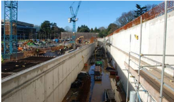
198 199 Figure 1: Construction site in February 2014. View 200 towards the West end where the tank had to be cut 201 deepest into the ground 202
