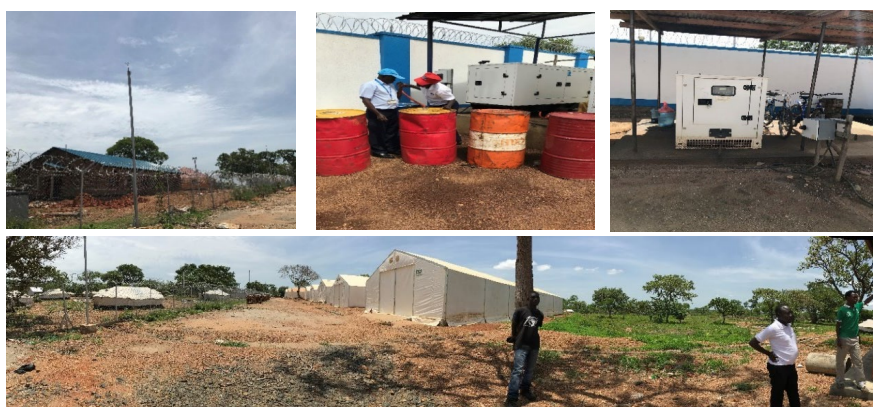
Figure 4 Bidi-bidi base camp secured fencing (top left), UNHCR staffs are checking a reported diesel fuel contamination issue (top middle), a 50kW diesel generator (top right) and relief storage facilities that require uninterrupted power supply (bottom).
