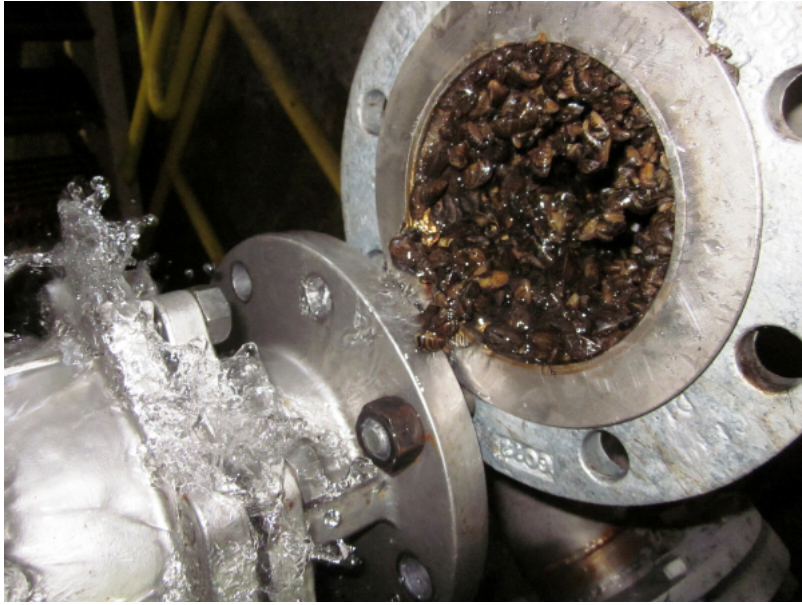
Figure 1.1: Extent of zebra mussel colonisation of intake pipe
