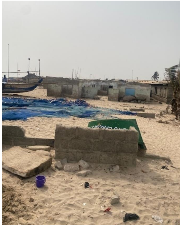
Figure 6.4 Damage to dwellings from flooding and erosion in Anyamam (S2). Damage resulted in the displacement of some households; however, despite some dwellings being partly submerged in sand, many continued to reside in their homes due to “place attachment”
