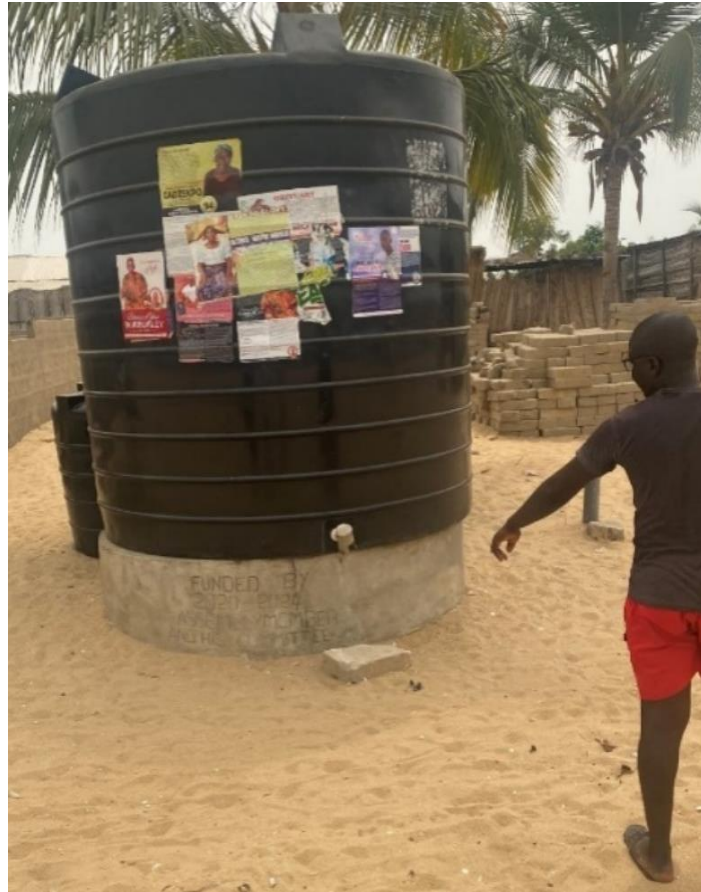
Figure 5.9 Piped water supply in Kedzi (S7), funded by the community assemblyman and their committee in 2020
