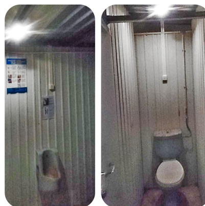
C Urinal (left) and toilet (right) powered by MFC electricity
