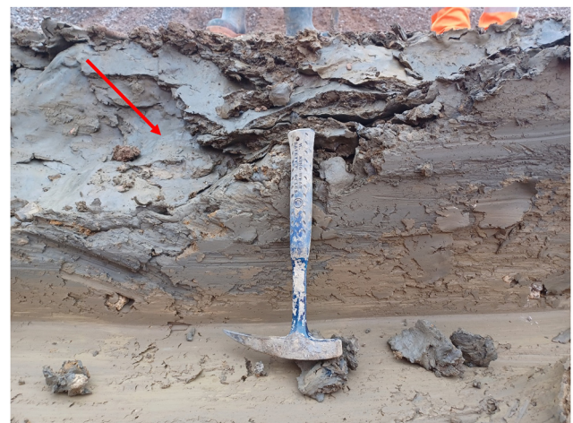
Fig. 9. Frequent shallowly becoming steeply dipping, undulose, closely spaced shears (Type 1) in head deposits at 0.6–0.8 m depth below original ground level in excavations near Waddesdon (WA), Buckinghamshire. The hammer is 330 mm long.
