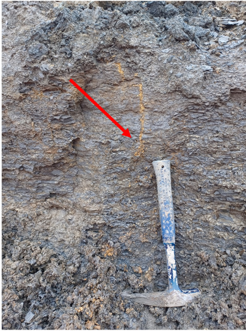
Fig. 12. Orange yellow silt and sand filled thin subvertical veins (Type 7 contraction cracks) in extremely weak mudstone (at c. 2.5 m below original ground level) become folded and irregular as they terminate in the overlying weathered clays of the Kimmeridge Clay Formation (Ancholme Group) in an excavation near Aylesbury (AY), Buckinghamshire. The hammer is 330 mm long.
