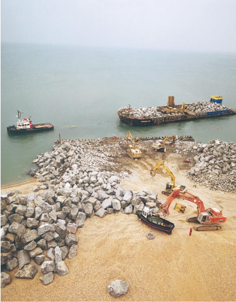
Fig. 5. The client paid for rock revetment based on weight of rock delivered
